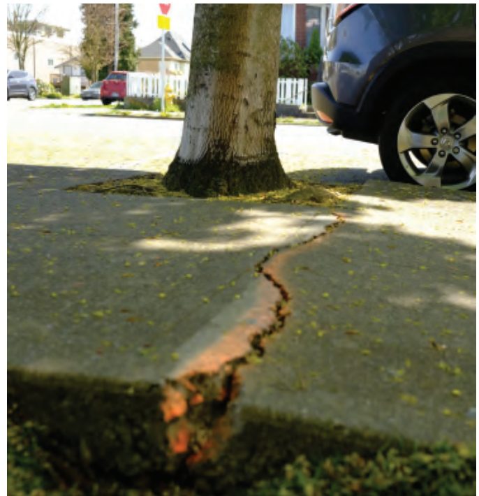
Tree roots lifting a sidewalk.
