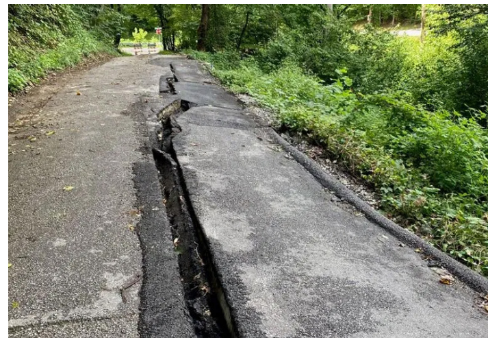
Rain events can overwhelm infrastructure, causing damage. Image Source: WCHS News
